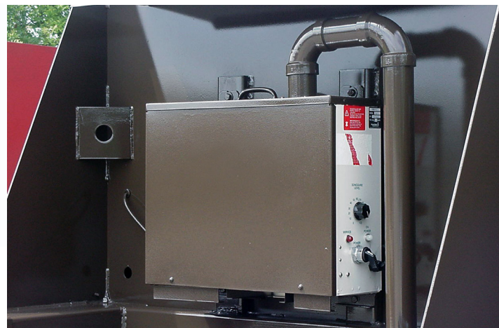
Marathon's Ozone Odor Control System installed on a Vert-I-Pack vertical compactor.
