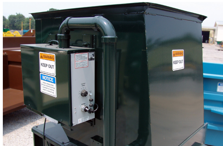
Marathon's Ozone Odor Control System installed on a Mini-Mac apartment compactor.
